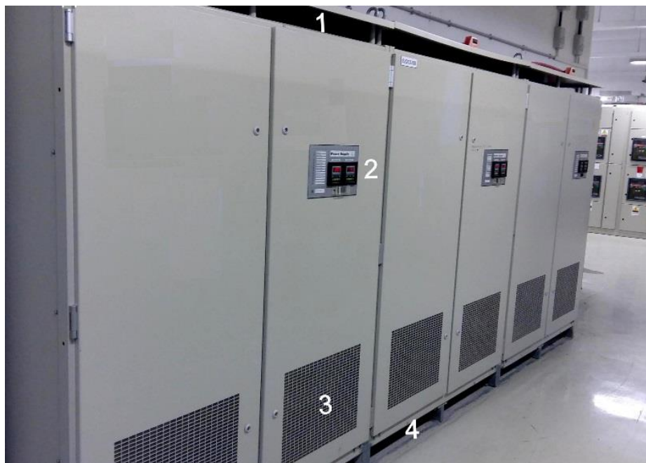
Figure 1: Design of power plant's BC. The figures indicate the “weaknesses” of cabinets that allow unobstructed access of HEMP inside the cabinet.
